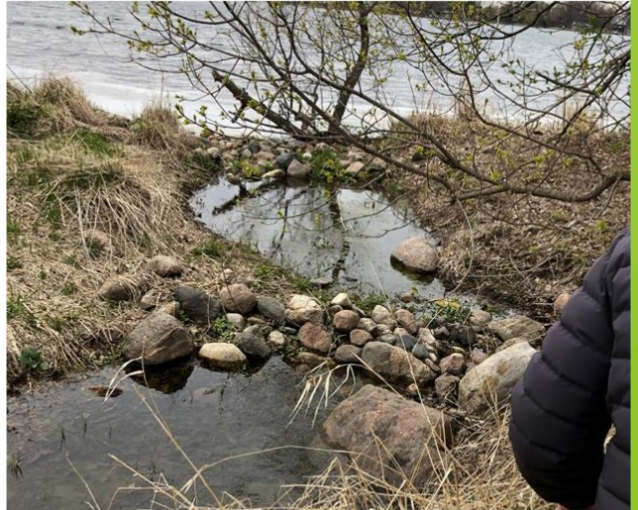
Figure 2 2021 Photograph of the Loose Rock Dam on Somers Lake (photo courtesy of the MNDNR)
